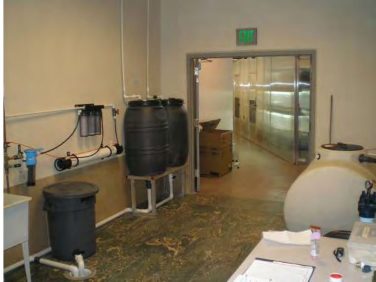
Figure 8. The building's water storage and central treatment station.
